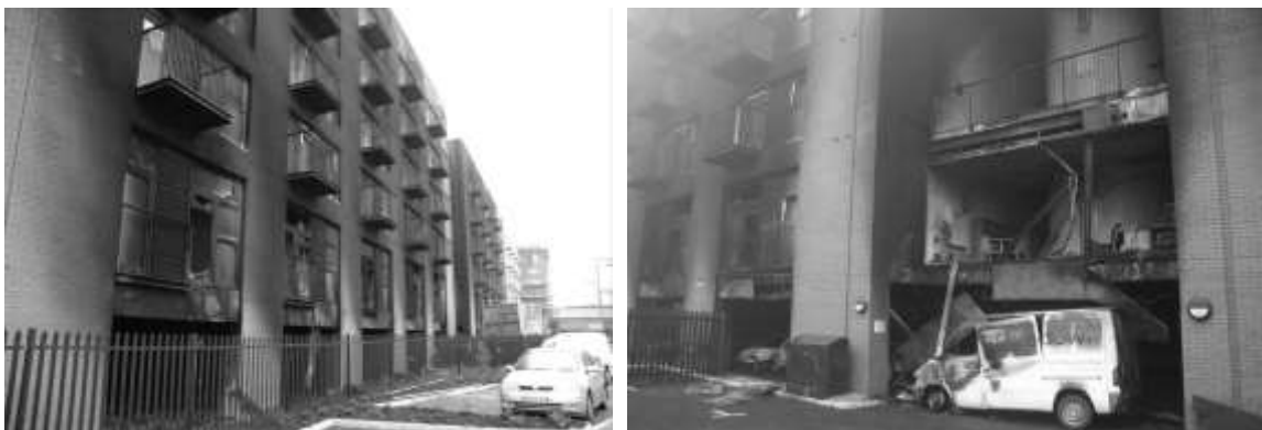
Figure 3 & 4 – example of the hazards of ventilation openings adjacent to a buildings facade
