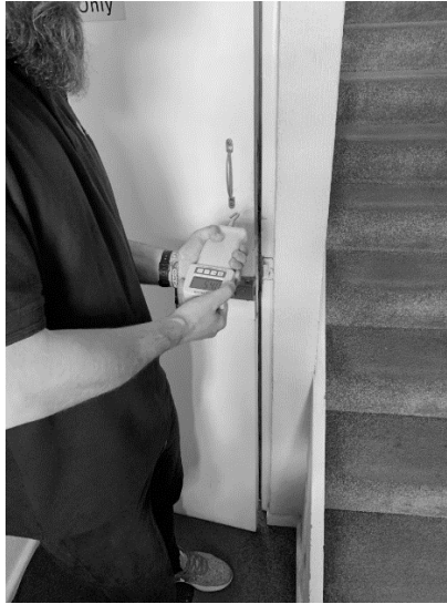
Figure 3 – It is important to always check the force required to open a door within escape routes to ensure compliance with regulations
